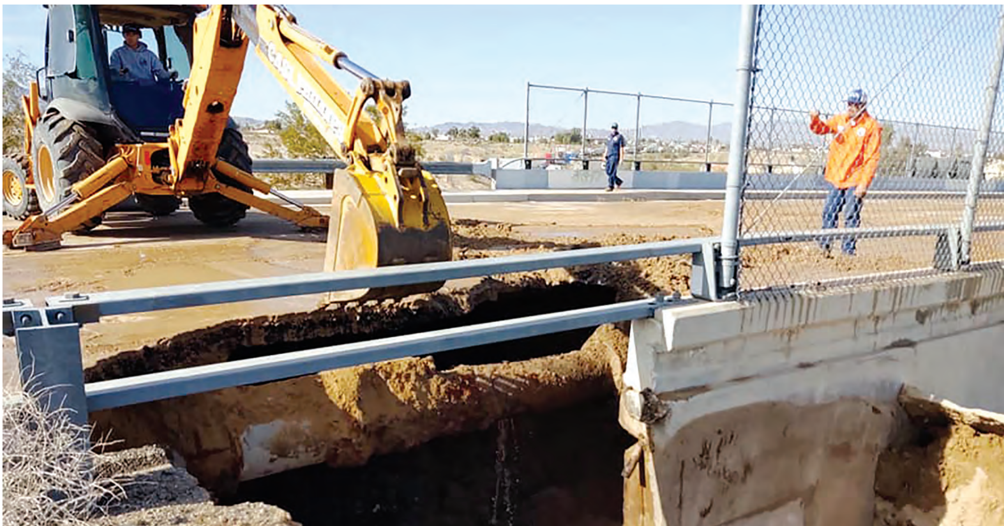
In January 2020, Needles' one pressurized water line to its reservoir burst under an Interstate 40 bridge, as shown above and at far right. Residents were alerted to conserve water and the state stepped in to help with the repair. However, that emergency plus 250 water leaks and the loss of two water wells last year, served as a wake-up call for city officials and residents as to just how dire their aging water infrastructure situation has become.
