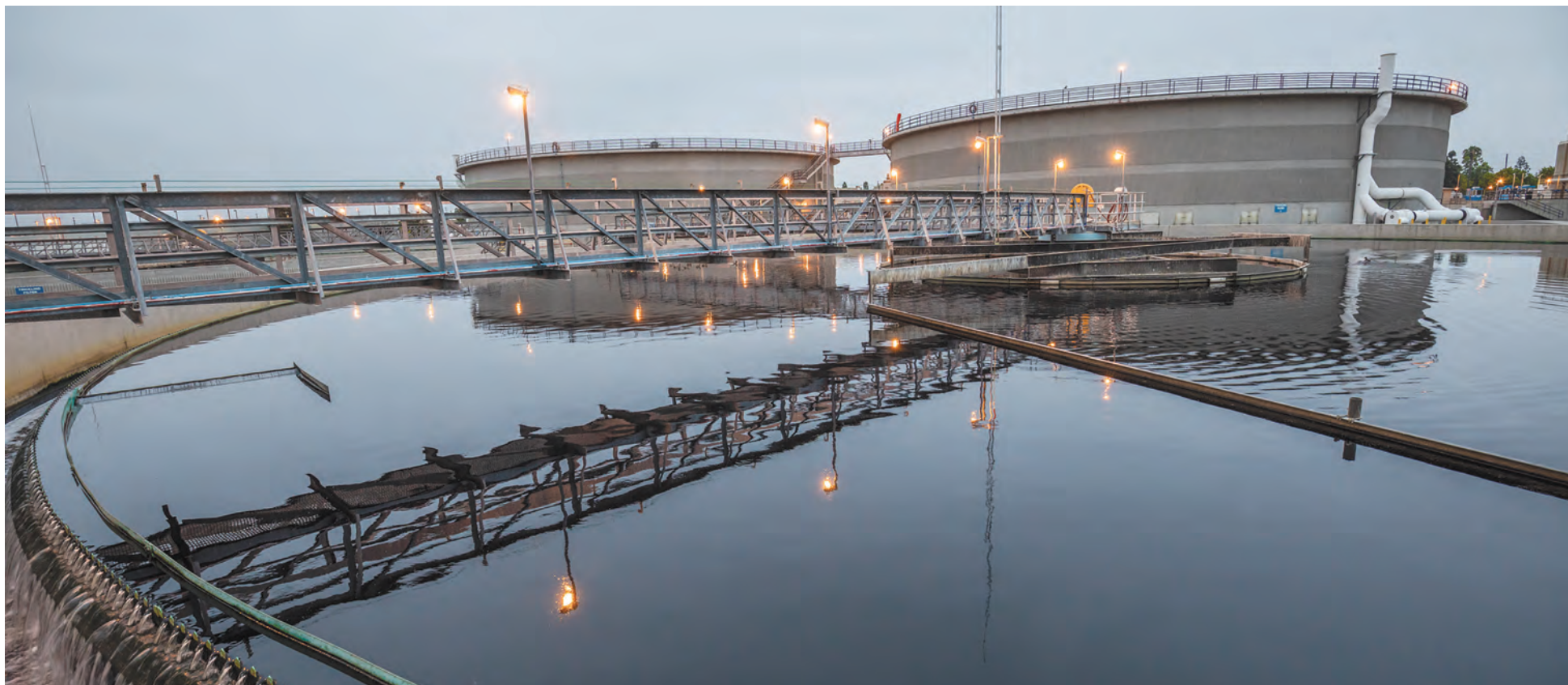
OC San's wastewater collection facilities include 388 miles of sewer pipes and 15 pump stations throughout the service area, and two 100-acre water resource recovery facilities located in Huntington Beach and Fountain Valley. Pictured above a secondary clarifier at Plant No. 1 in Fountain Valley.
