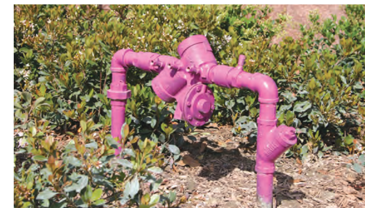
Purple piping refers to lines designated for recycled water, which is treated to a level suitable for irrigation and industrial use, but not for drinking.
