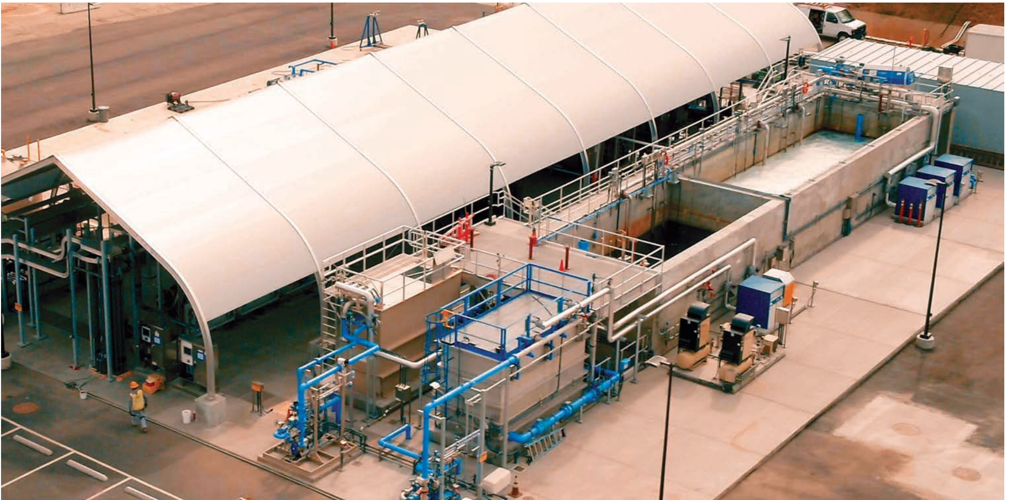
Located in Carson, this demonstration facility purifies 500,000 gallons of treated wastewater per day by using membrane bioreactors, reverse osmosis and ultraviolet light to remove bacteria, minerals and other chemicals. A full-scale facility would make the region less dependent on imported water. Photos courtesy of the Metropolitan Water District of Southern California
